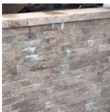
Mineral deposits on a wall installation
